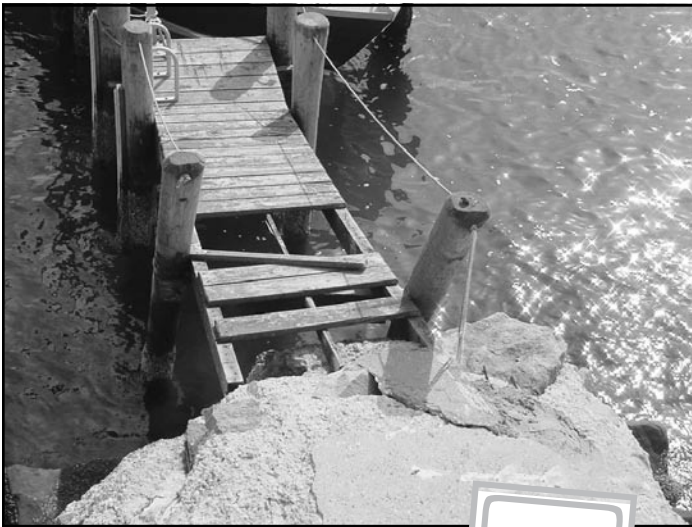
Damage to dock
