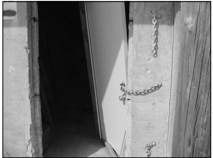
Entrance door and frame stove in
